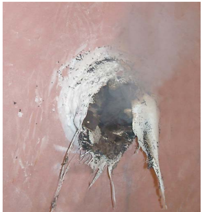
A Pipe Penetration Successfully Sealed by a Fire Collar
