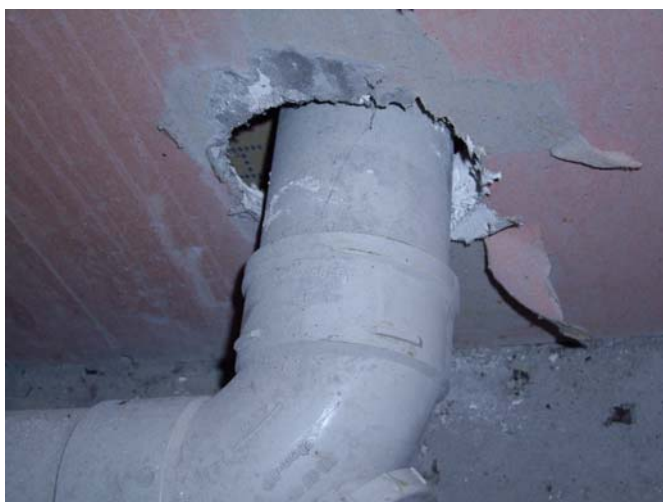
Fire Rating Compromised by Pipe Penetration
